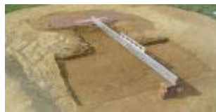
Excavate the landing area and be 10" wider and longer than the longest stride of your pitchers. Blocks should be within a 1/2" of the surface.
