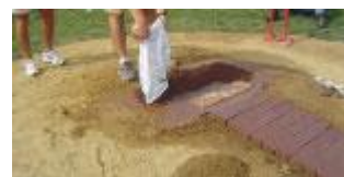
Apply a thin layer of Professional Mound Clay (match color to blocks), moisten and tamp.
