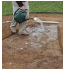
STEP 2: Moisten the bottom of the hole with water. Add an inch of Turface Professional Mound Clay with a rake, cut into the soil for proper bonding. Tamp firmly. Lightly moisten but do not drown and tamp again.
