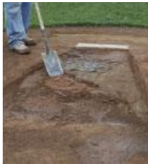
STEP 1: Excavate the front slope of your mound to a 4" to 6" depth. Batter's boxes and catcher's box to a 4" depth.
