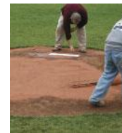
STEP 5: Add a final coating of water on the Turface Professional Mound Clay areas once all grades and slopes are set and rolled. Finally, topdress all Turface Professional Mound Clay areas with your infield mix and conditioner to match the color of your infield.
